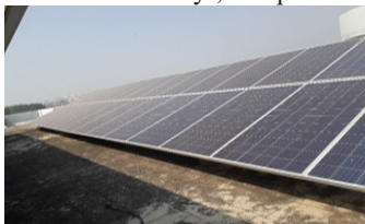
Fig. 1: Commercial sized solar arrays installed.
