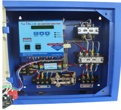
Fig.4.5 HP PANEL BOARD
